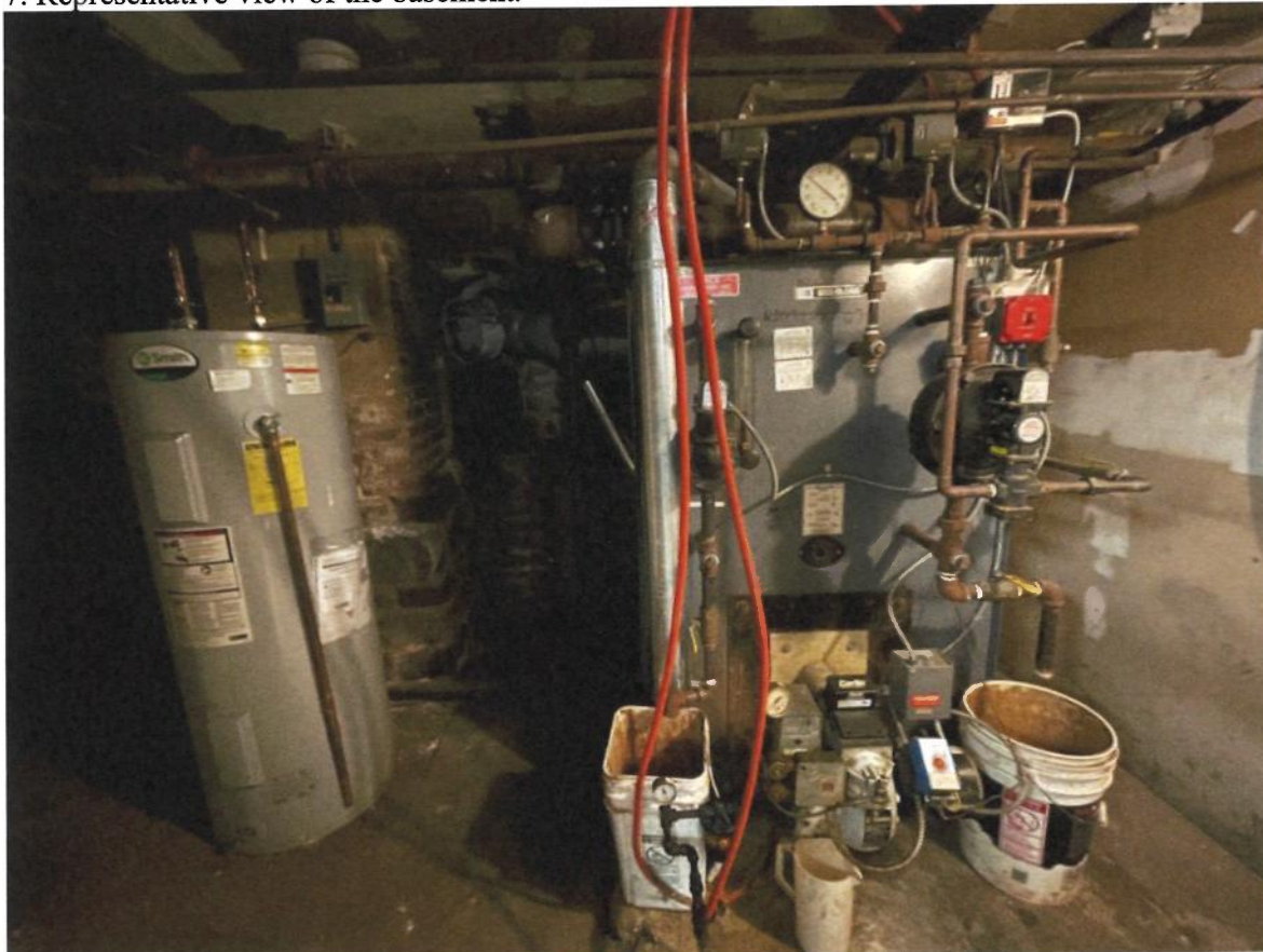
8. Representative view of the boiler room.
